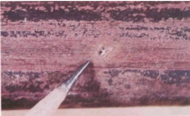
Fig. 12. Oxygen pitting attack on copper tube.
