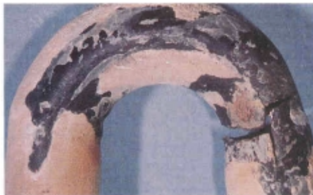
Fig. 5. Thermal fatigue failure in U bend.
