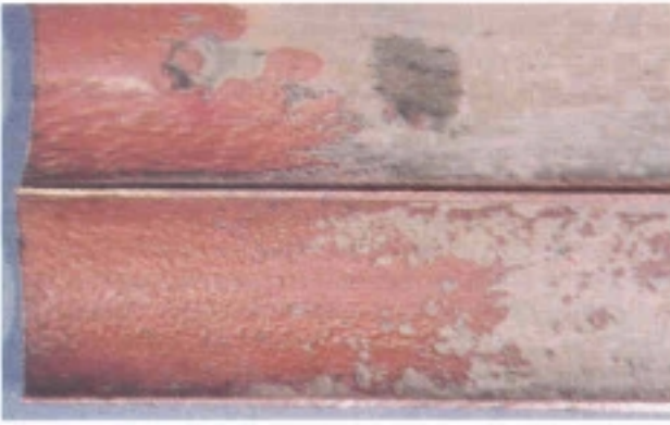
Fig. 19. Erosion-corrosion attack on tube.
